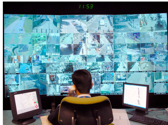
Figure 3: Town Centre Camera Surveillance Control Room. Image Source: www.barco.com
