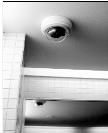
Figure 4: rest room camera
